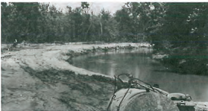
Figure 16. Debris and sediment removal was accomplished by working from one side of the stream. Selected trees were cleared to allow equipment access and operation. Trees have now grown back on the cleared side.
