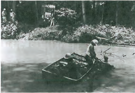
Figure 14. Hand labor crew in boat hooking cable to log. The small crawler tractor with winch will pull the log from the stream. Small equipment can be carefully maneuvered through the floodplain forest causing little damage.
