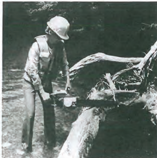
Figure 13. Chainsaw being used to cut log so that it can be pulled with small hand winch and repositioned along stream bank.
