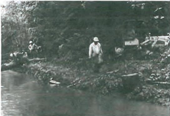
Figure 15. Hand labor crew hooking cable to log to be pulled from stream by small crawler tractor with winch. Only a narrow work zone along the stream was disturbed because of the small equipment. Note stump left in place to stabilize bank.
